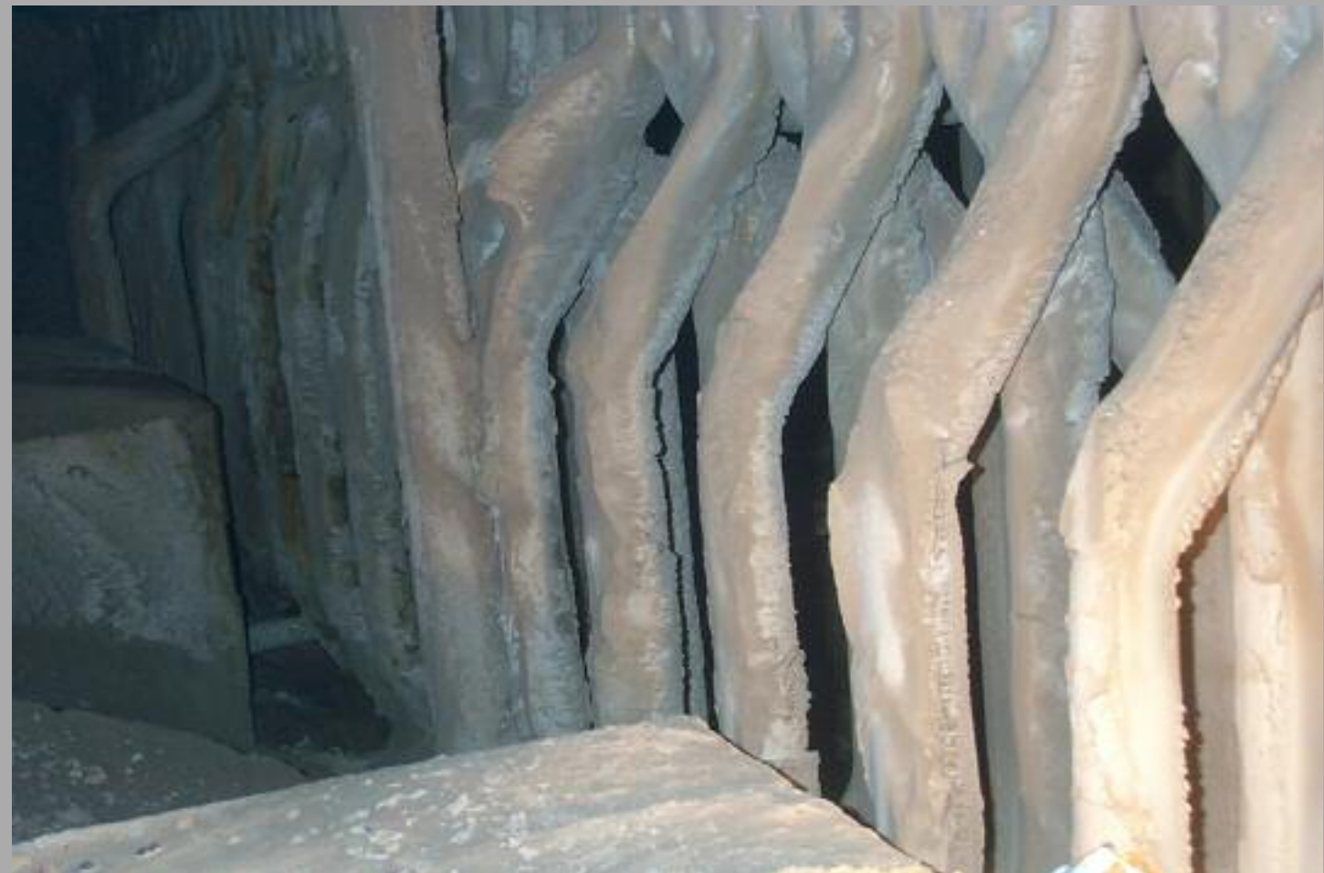
Boiler exit screen – 76mm O.D. tubes
