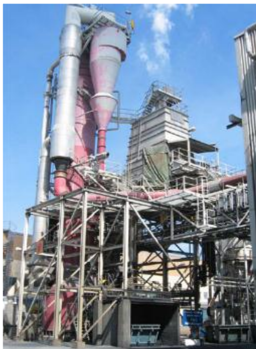
CFB Metso, wood, Varo (Swe), co-firing lime kiln 35 MW th_biomass
