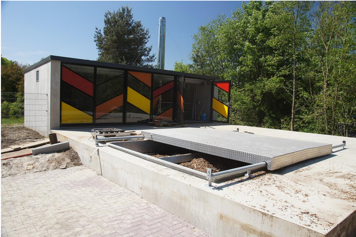
Figure 3: The biomass plant in the centre of the village of Marum, with underground fuel storage and mostly underground boiler room.
